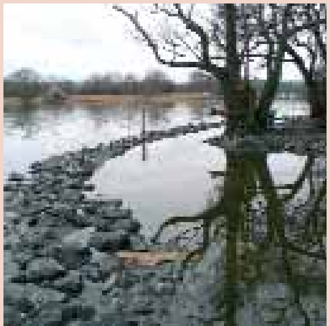
Above and opposite: Work to stabilize the crannog in progress. Opposite, top: The new visitor centre.
